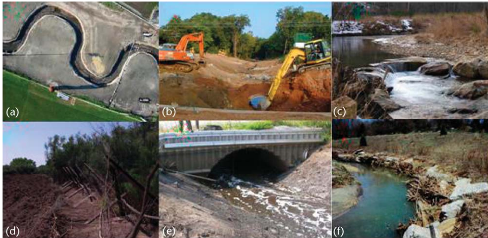
Figure 2 Photographs of common restoration practices: (a) an urban ‘daylighting’ project in which a formerly piped stream is uncovered; (b) installation of a natural channel design project; (c) a rock weir structure installed for grade control within a natural channel design project; (d) removal of invasive species from riparian areas; (e) improved, large diameter road culverts installed to allow fish passage and (f) bank stabilization with root wads and coir fibre matting. Photo credits: (a) Chris Benton, (b) Barbara Doll, (c) Emily Bernhardt, (d) Jennifer Follstad Shah, (e) Marcelo Ardón and (f) Emily Bernhardt.
